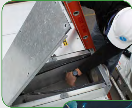
Inlet strainer inspection for Series 1500
